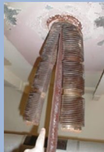
3. This stainless steel bellows failed because expansion was greater than predicted (above)
