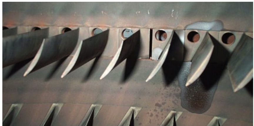
1. Gaps between adjacent blades occur when shims wear and fall into the flow stream, causing foreign object damage
