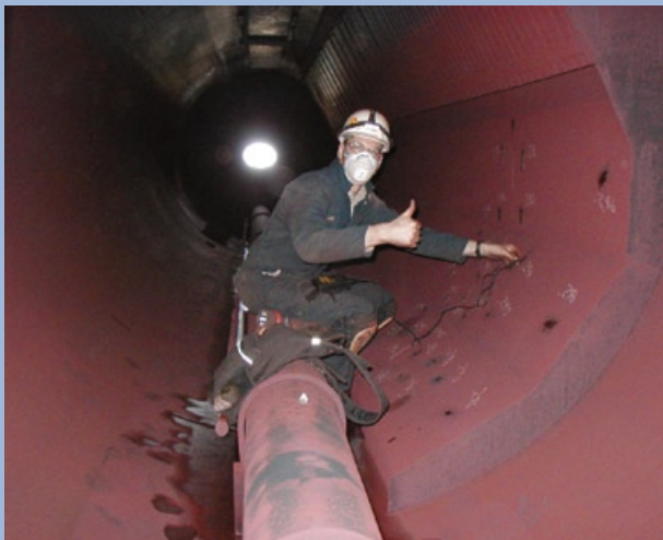
2. Ultrasonic thickness testing revealed no problems in this low-pressure drum, but does that mean the rest of the boiler is fine?
