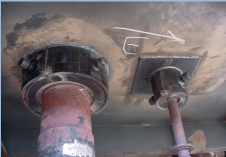
5. Retrofit pipe penetration seal designed by HRST is said to be increasingly popular
