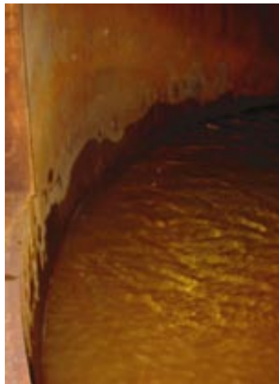
17. Inspector found approximately 8 in. of standing water in stack base
