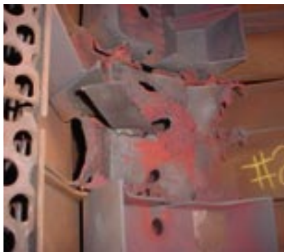
9. Oxidized burner components require replacement
