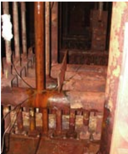
13. Leakage through riser penetration reaches tube bundle below
