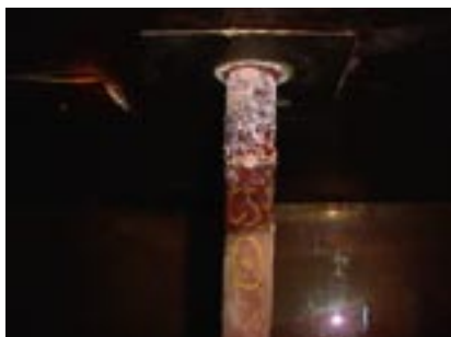
12. Rainwater leaking in through penetration seal corroded economizer vent pipe
