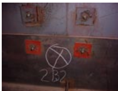
11. Conspicuous color changes in liner system help identify problem
