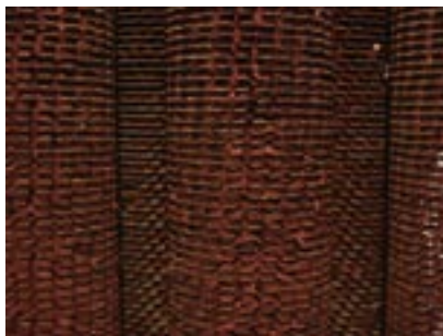
6. Scale between fins is a consequence of offline corrosion
