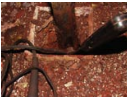
14. Measure thickness of drain-pipe wall to determine corrosion rate. Access is easier if penetration seal is removed from casing exterior
