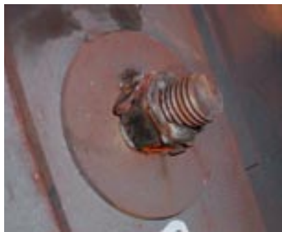
10. Incorrect material use was cause of high-temperature corrosion here
