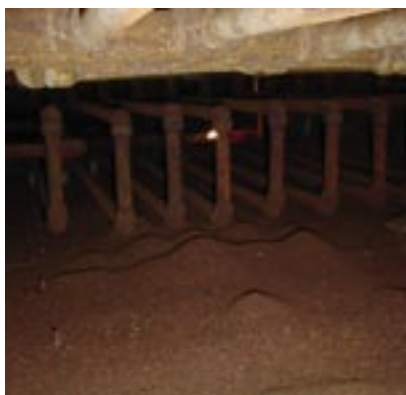
7. Offline corrosion causes debris to accumulate in lower crawl-space
