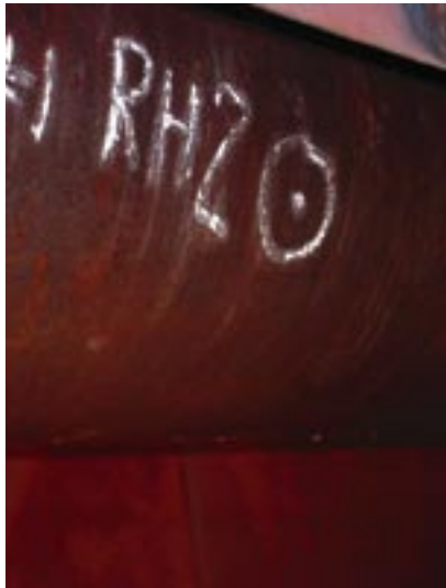
5. Condensate drips from lower reheater header while unit is shut down
