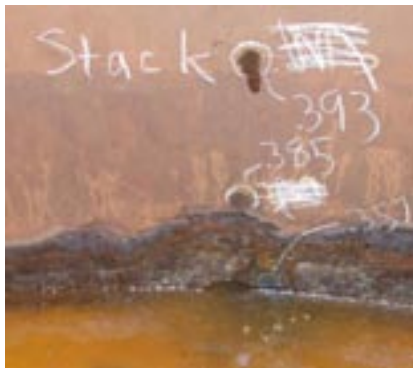
16. Corroded stack base. Numbers on wall are ultrasonic thickness measurements. Material wastage is significant
